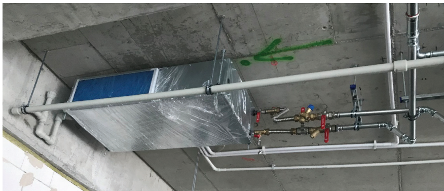
FIGURE 6. The heat pump (WLHP) connected to the water installation by the pipe system with the control valve, the sieve filter and shut off valves (author: Dorota Leciej-Pirczewska)
