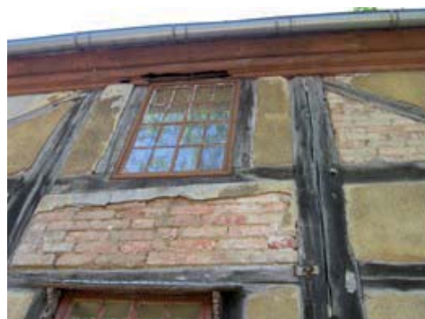
FIGURE 3. Northern elevation – fragment. The corroded wooden post and beam structure. Loose brick connections, missing plaster. Corroded attached canopies over the ground-floor window
