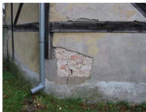
FIGURE 6. Fragment of the south-western elevation. Cracking of the plinth in the corner between the south-western wall, missing plaster, cut-out fragment of post
