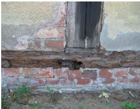
FIGURE 4. Northern elevation. Corroded ground beam, loosened connections of plinth brick, missing areas of plaster. Between the post and the corroded and crushed ground beam, the crevice is filled with an insert from boards
