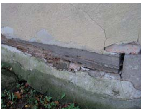
FIGURE 5. North-western elevation – fragment. The corroded and compressed ground beam. Damp foundation plinth
