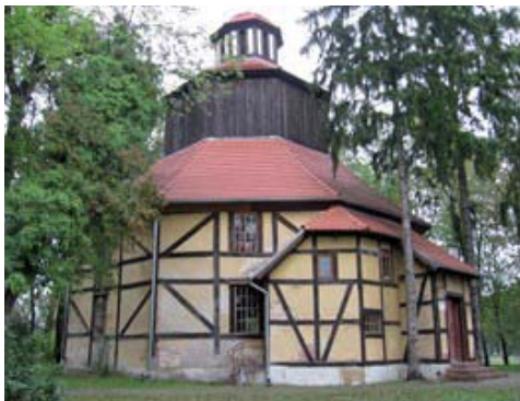
FIGURE 1. The south-western elevation. Damaged and damp foundation plinth, corroded wooden structure, significant missing areas of plaster in the masonry wall filling the post and beam structure
