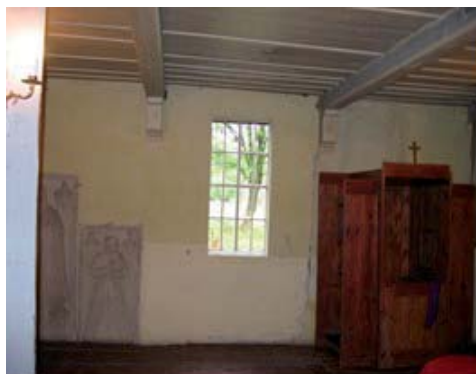
FIGURE 7. Inside part of the north-eastern wall. Vertical cracks of the wall along the posts
