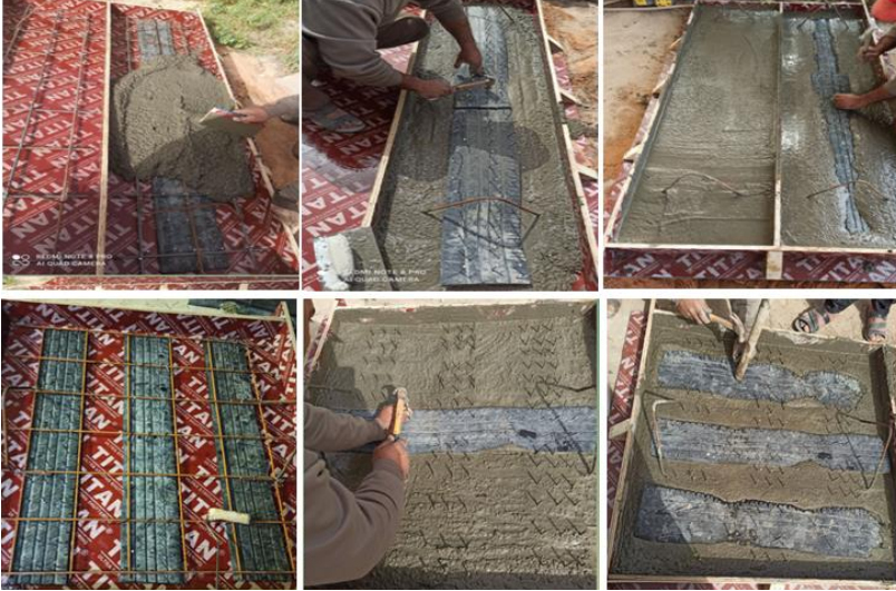
FIGURE 4. Reinforcement and DTS fixing processes and concrete casting for the RCOWS and RCTWS models
